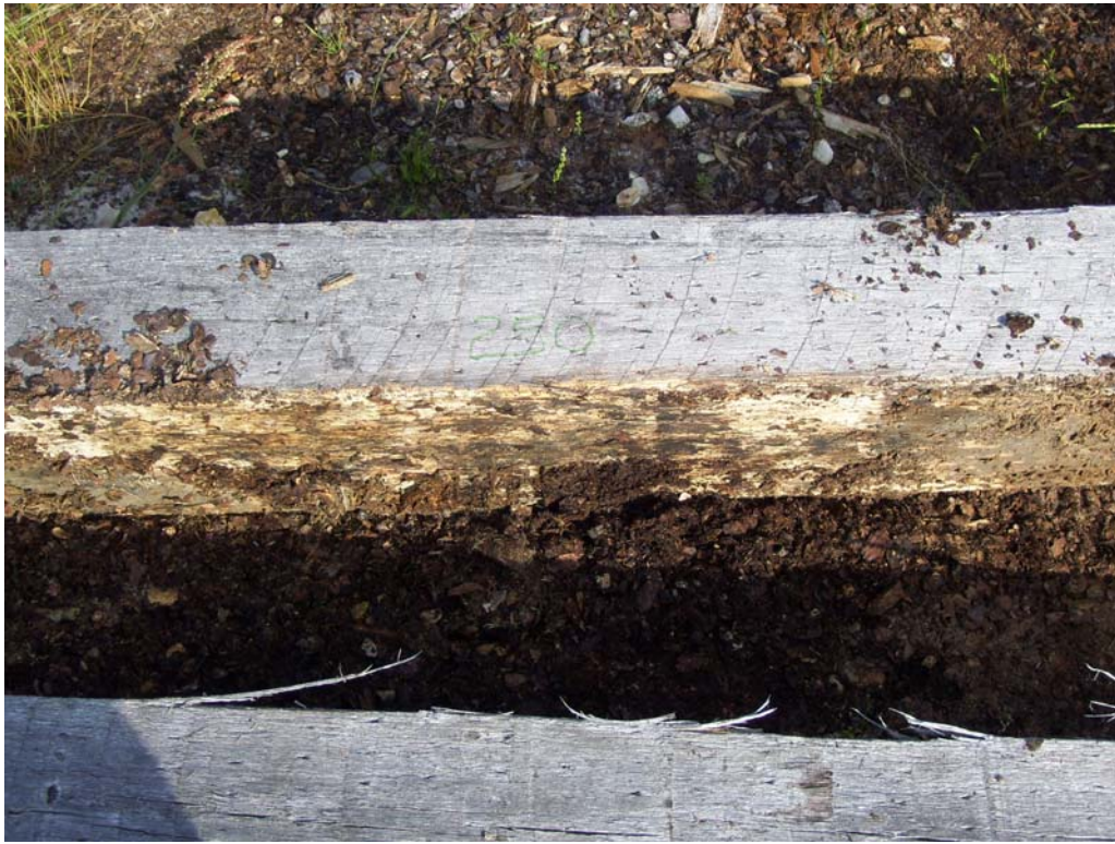
Figure 8 - Tie #250 with slight decay.
