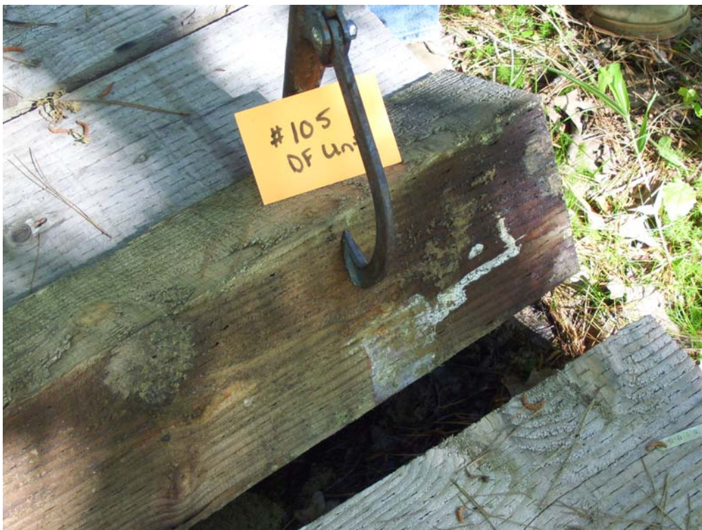
Figure 3 - Tie #105 showing trace amounts of decay.
