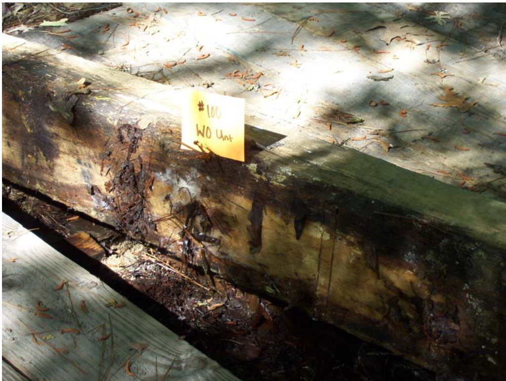
Figure 5 - Tie #100 (white oak/untreated) showing signs of decay.
