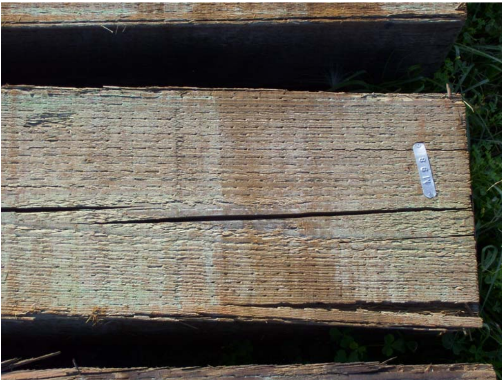
Figure 7 - Tie #98 beginning to check.
