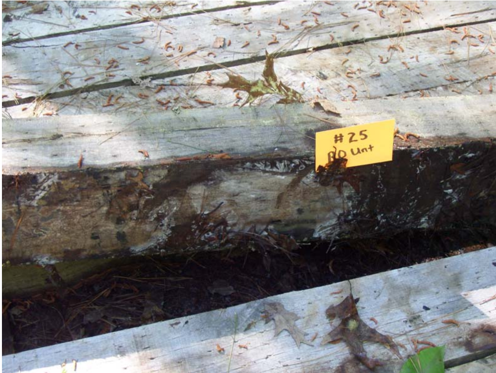
Figure 4 - Tie #25 (untreated red oak) with signs of decay.
